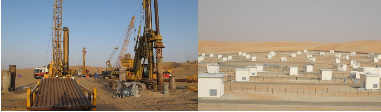
Figure 4. Construction of project infrastructure (left) and recovery and monitoring wells (right) (photo: M. A. Dawoud).
