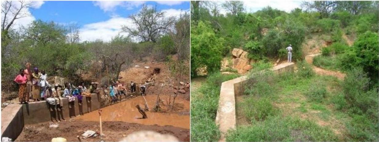
Figure 2. Sand dam in Kitui right after construction (left) and vegetation restoration of a sand dam after a few years in operation (right) (photos: S. de Wildt).
